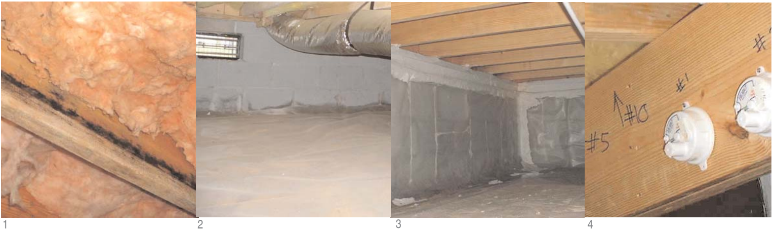
Photo one: Builders and homeowners are increasingly concerned about crawl space mold stains and odors.
